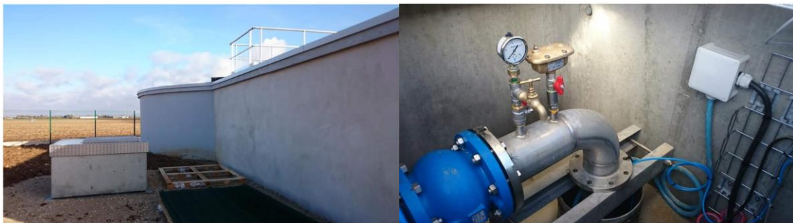
Figure 16. Installations de surface F2
